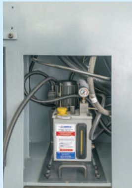
PLC programmable controlled Auto lubrication system for periodic and desired Quantity lubrication.
